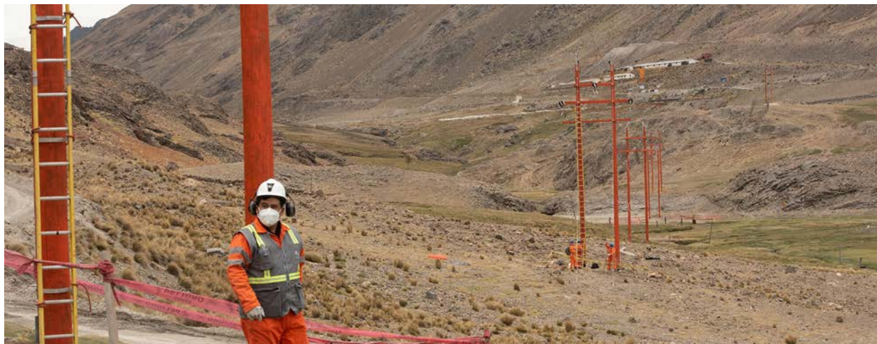
▼ Caylloma power lines
